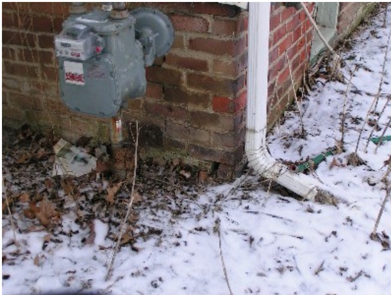
PICTURE 8 - foundation brick needs tuck pointing
