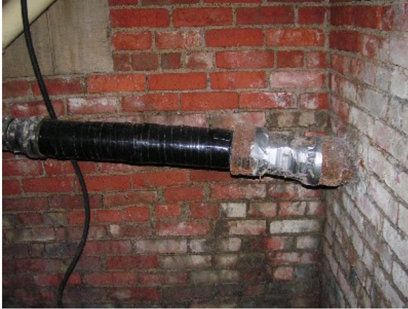
PICTURE 1 - sanitary discharge with duct tape
