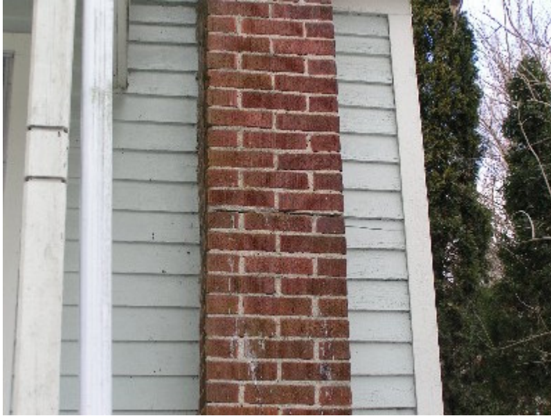
PICTURE 12 - crack in north chimney
