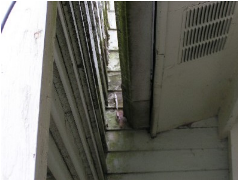
PICTURE 13 - rotted wood between north porch and house
