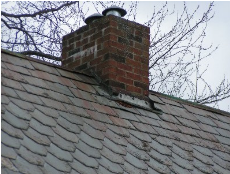
PICTURE 6 - flashing on main chimney
