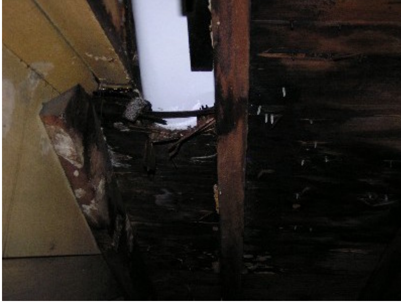
PICTURE 2 - north attic attach job---hole
